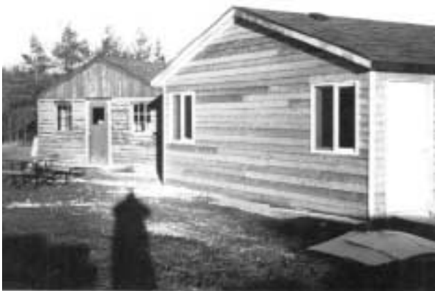
Anniversary Lodge under construction in front of Spectator Lodge just prior to its demolition - 1997
